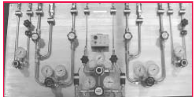
High purity changeover manifold with distribution
